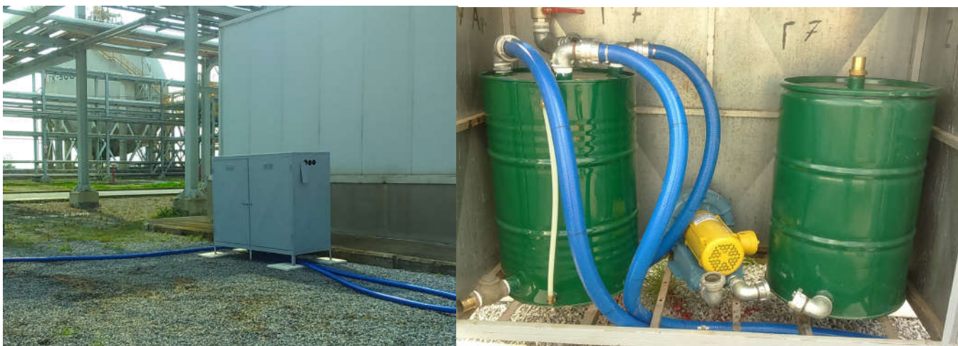
Photos 1 and 2: Metallic protective box which will enclose each SVE/Biosparging system (also shown the air/water separator bin and also the activated carbon bin)
