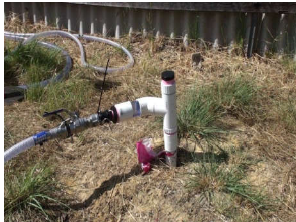
Picture 2a: In situ chemical Oxidation (ISCO). Injection Method : By means of existing injections wells (permanent wells)
